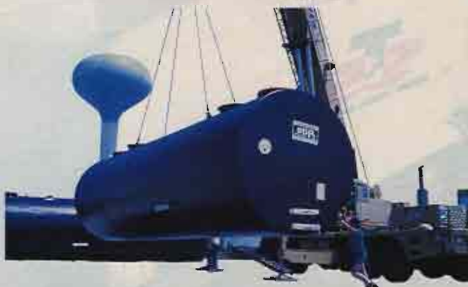
Replacing an existing three-tank facility with three-USTs will cost roughly between $80,000 to $100,000, says EPA.
